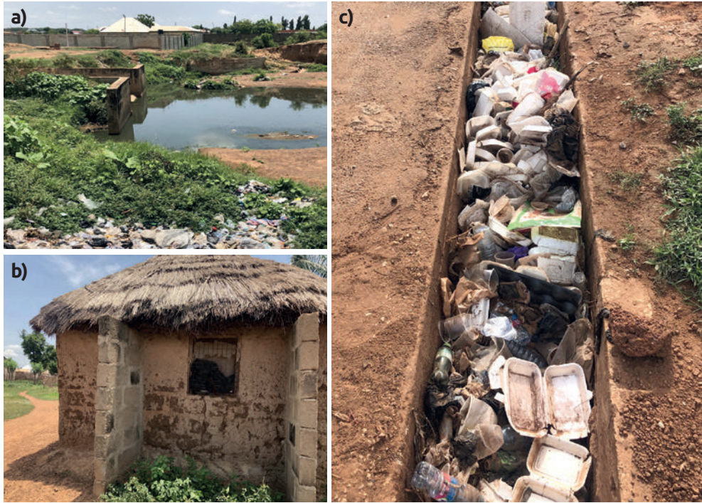
Figure 2: a) A city-level storm drain that stops abruptly in a poor community. b) Piers of concrete blocks added to a mud house to increase its resilience to flooding. c) A roadside storm drain blocked with solid waste rendering it ineffective. (Credit: Ben Howard and Cynthia Awuni)
